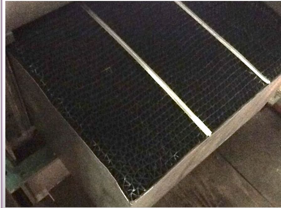
Top View of Module Removed for inspection
